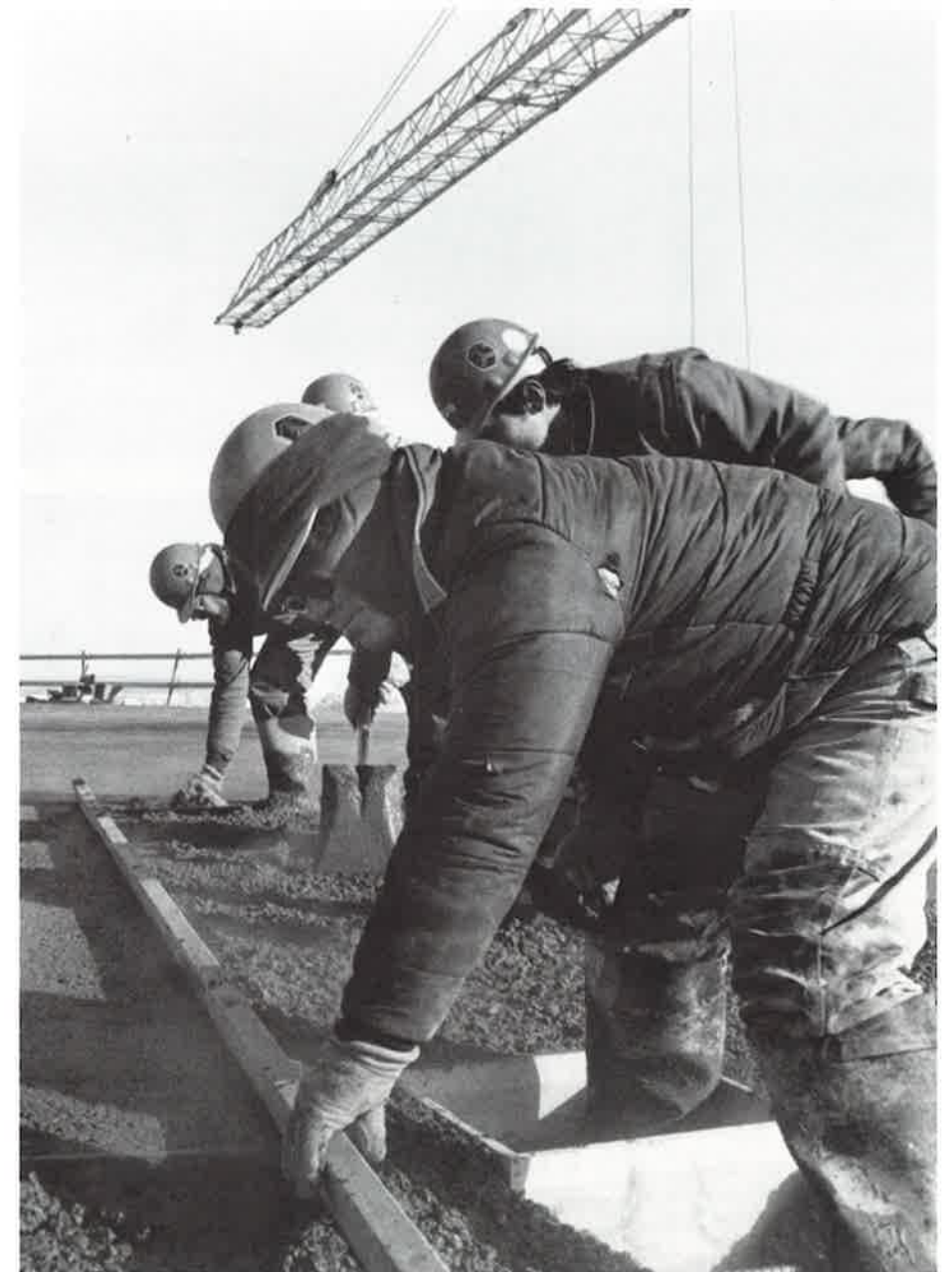
Workers poured the concrete roof of the new CSD headquarters building in late January. See pages 1, 4 and 5 for a quiz about Sperry's other facilities.
