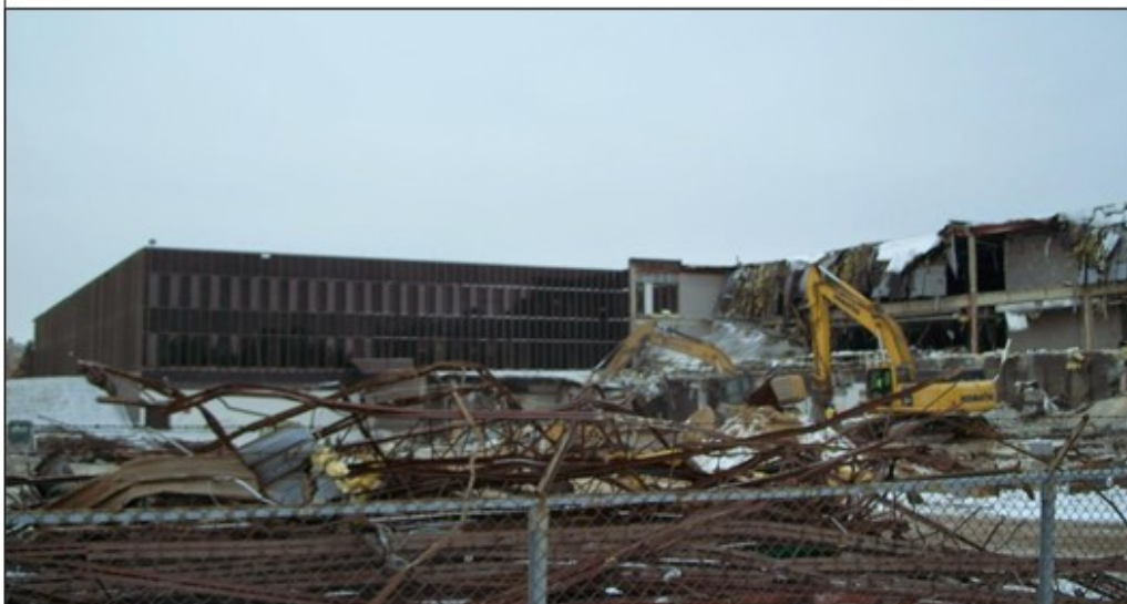
Below: The demolition of the Lockheed Martin plant on the corner of Pilot Knob and Yankee Doodle roads in Eagan dated March 2015. It is currently being developed by CSM Corporation as a 434,000 square foot retail and office center which will be known as "Central Park Commons." Image courtesy of Tim Johnson.
