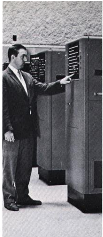
A portion of the system's control units.
